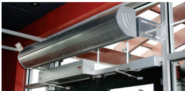
Air door at the main entrance provides comfort and heating cost savings.
