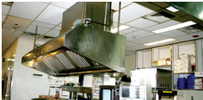
Demand control kitchen ventilation ensures fans in this hood respond to actual stove use.
